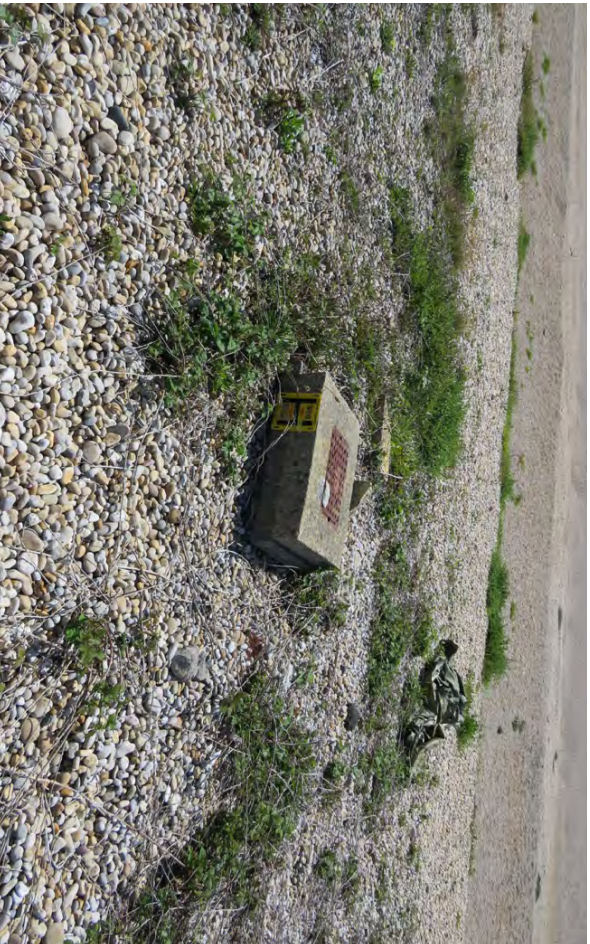
Photo 15: Evidence of utilities within vegetated coastal shingle habitat within Chesil and the Fleet SAC.
